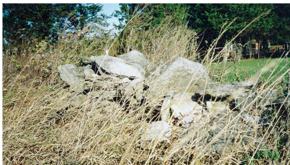
Pentland Fence in need of restoration
